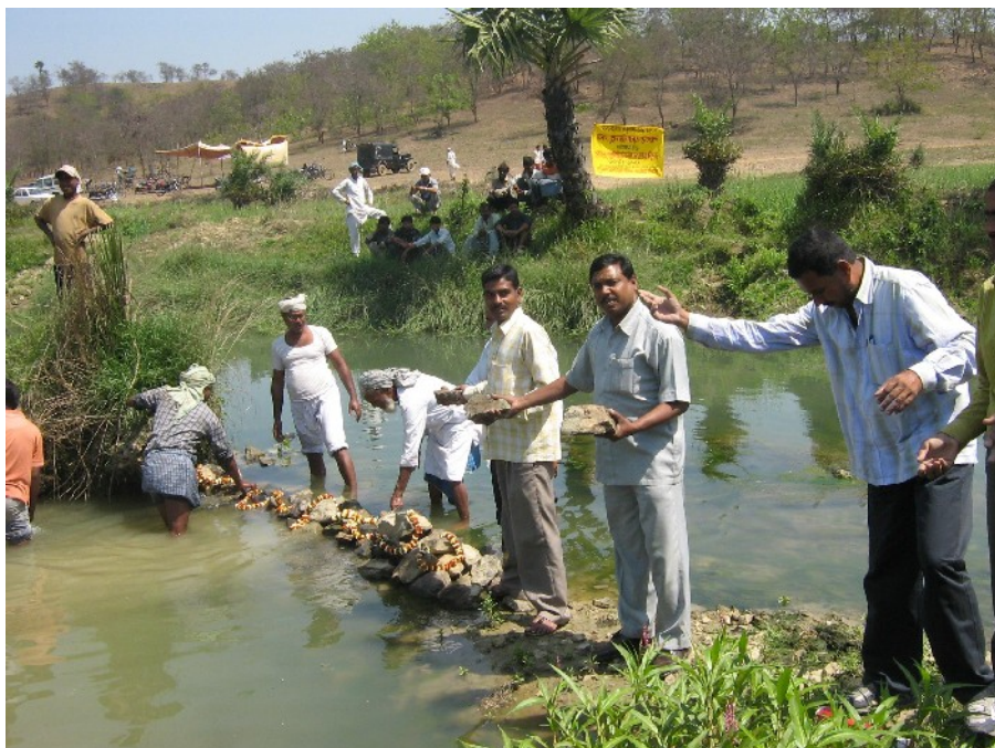
Repairing and mending a pyne by a voluntary effort in progress in Gaya district.
